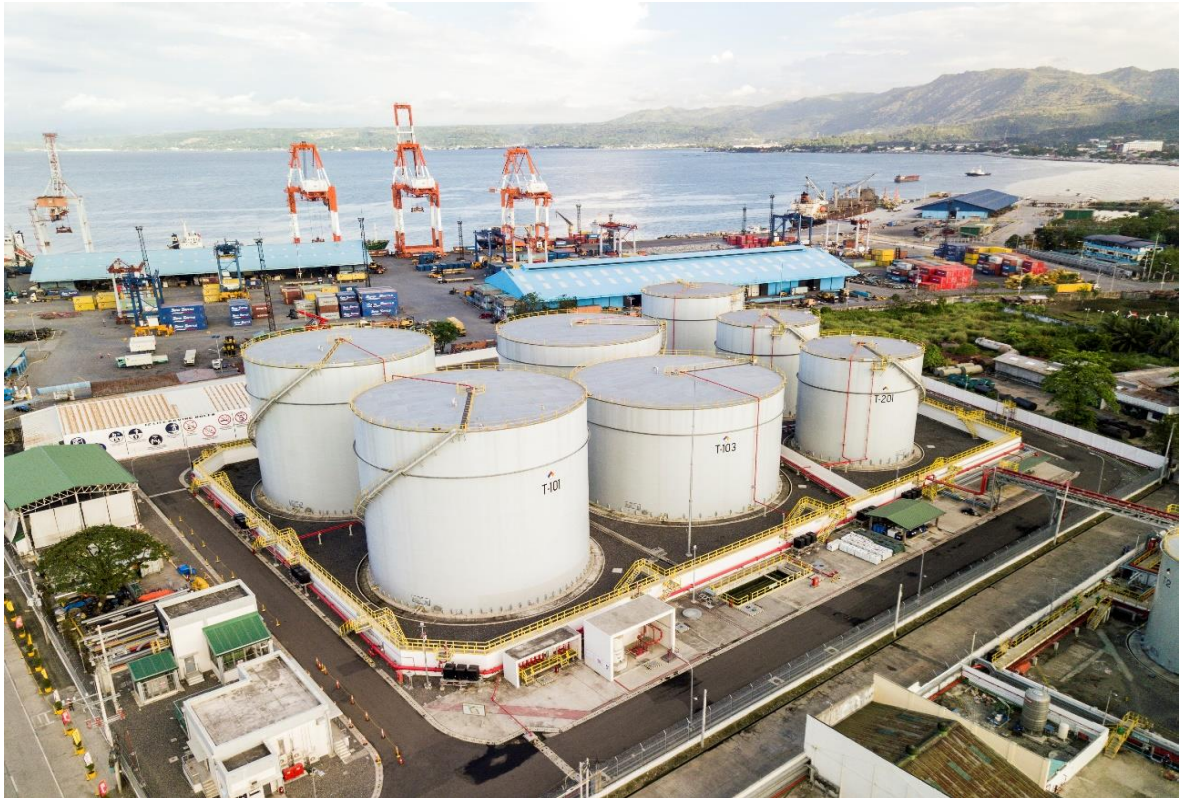
Fuel storage tanks at Shell's Northern Mindanao Import Facility
